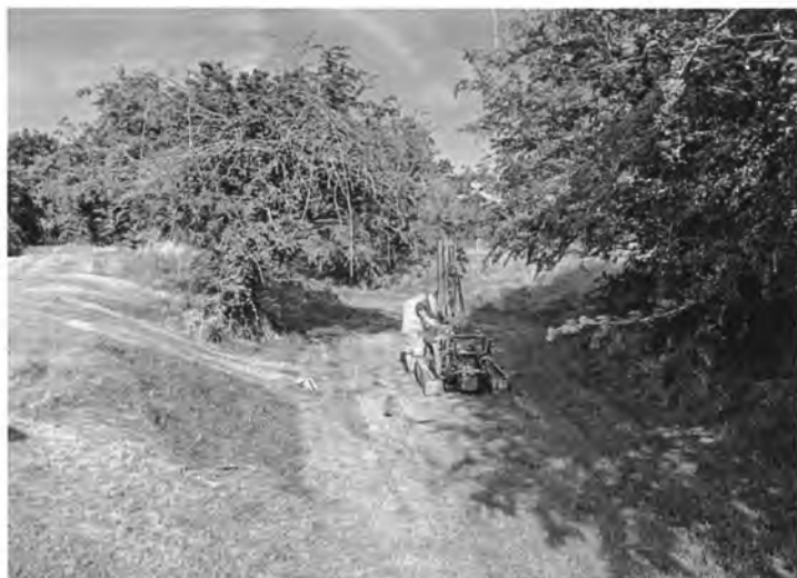
Plate: Borehole drilling under way in the centre of the Burton Lodge ditch.
